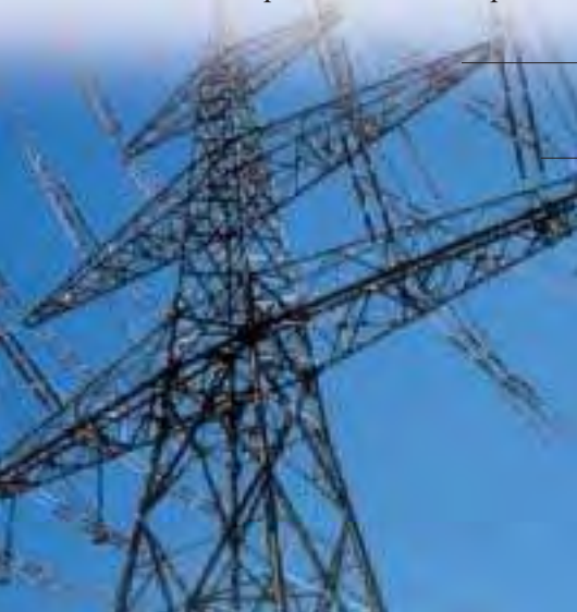
Steel pylon strong enough to support the cables
