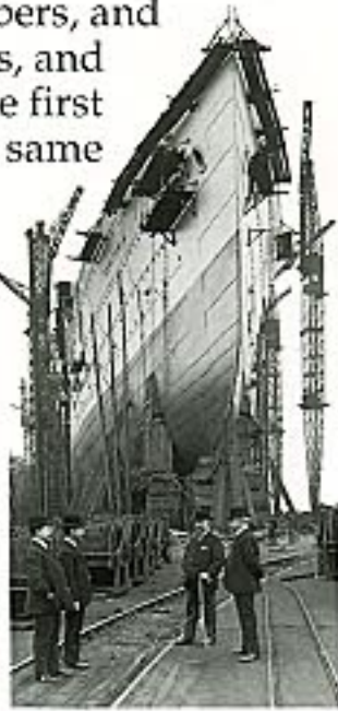
ON THE STOCKS To allow easy access and an easy launch, the hull of a ship under construction is held in place by wooden supports called stocks. This picture shows the luxurious liner the Aquitania (pp. 54–57) in 1913. She was launched, stern first, into the River Clyde in Scotland a few weeks later.
