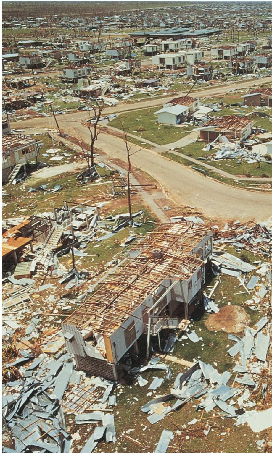
Hurricane David's powerful winds lifted this plane into the air, then deposited it on top of a hangar
