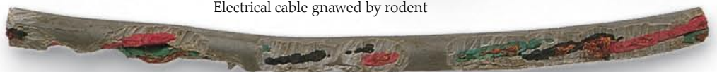
POWER CUTS Rats and mice may gnaw at electrical cables to find out what is inside. This can have consequences. Sometimes the animal is electrocuted. Fires and power cuts have been started by such "innocent" rodent behavior.
