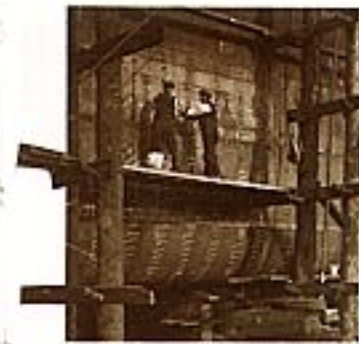
RED-HOT RIVETS These men are fastening hull plates together. Red-hot rivets are hammered through the drilled plates. A man on the inside of the hull then flattens out the rivet ends to stop them from coming out.
