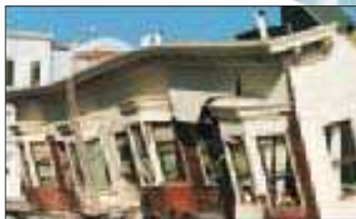
The 1989 earthquake struck the Santa Cruz Mountains in central California.
