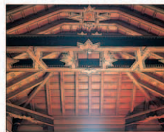
Cedar ceilings with geometric patterns, called alfarjes , were common in the 16th century.
