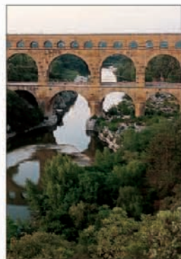
The Pont du Gard, outside Nîmes, a major feat of Roman engineering
