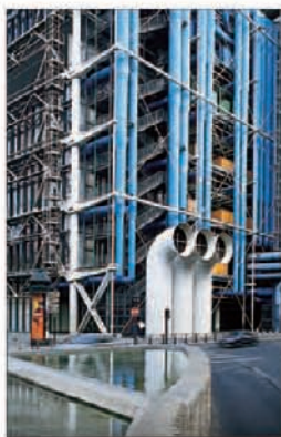
Pipes and ducts on the outside of the Centre Pompidou
