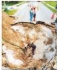
City workers surveying a sinkhole in the middle of a road
