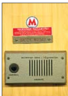
Emergency intercom to driver
