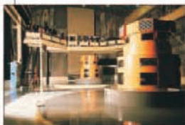
Underground machine hall
