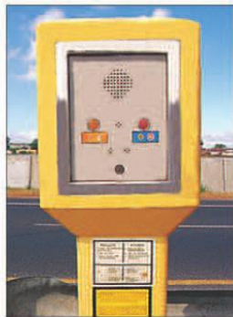
Emergency telephones are sited on some highways
