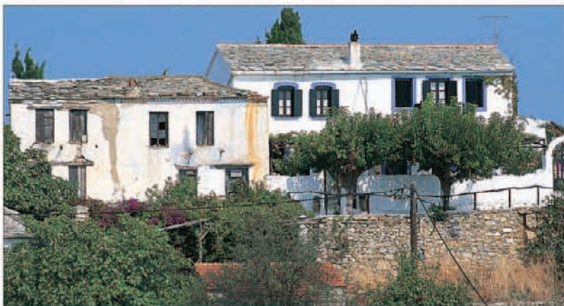
Two of the old houses in Palaiá Alónnisos in the process of restoration
