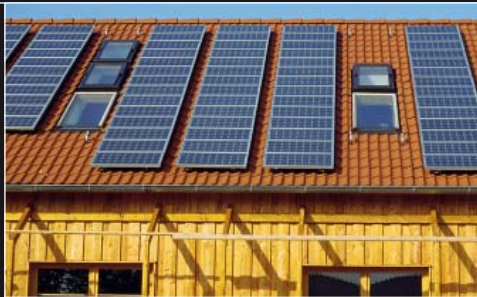
Photovoltaic panels on house roof
