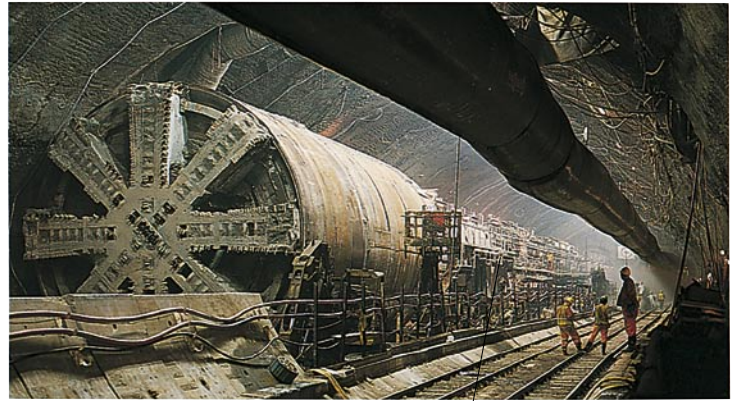
Machine carries two railroad tracks, nine computers, and ducts for air and water
