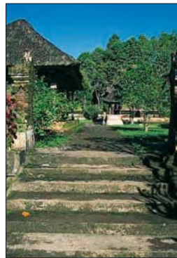
Steps to temple hindering wheelchair access
