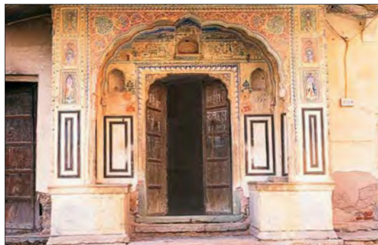
Faded wall paintings outside the palace at Bagru
