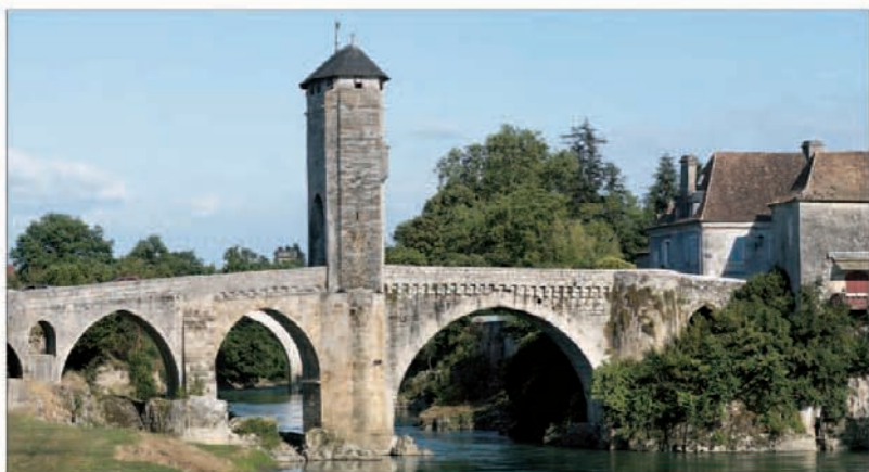
Pont Vieux, with its keep, over the Gave de Pau at Orthez
