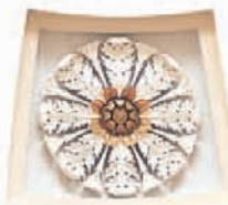
Pump Room detail, Cheltenham
