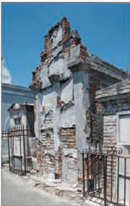
Creole family mausoleum, fallen into disrepair
