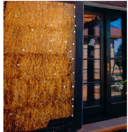
A wooden frame built with bale-sized spaces between the uprights is the perfect support.
